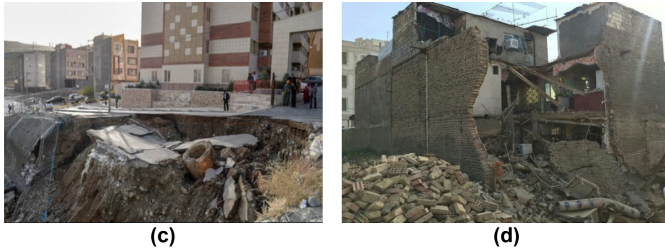
Fig. 4 - Excavation accidents in Tehran: (a) Talegani Street, Tehran, 2019; (b) A. Kashain Street, Tehran, 2021; (c) Saadatabad Province, Tehran, 2016; (d) West of Tehran, 2018
