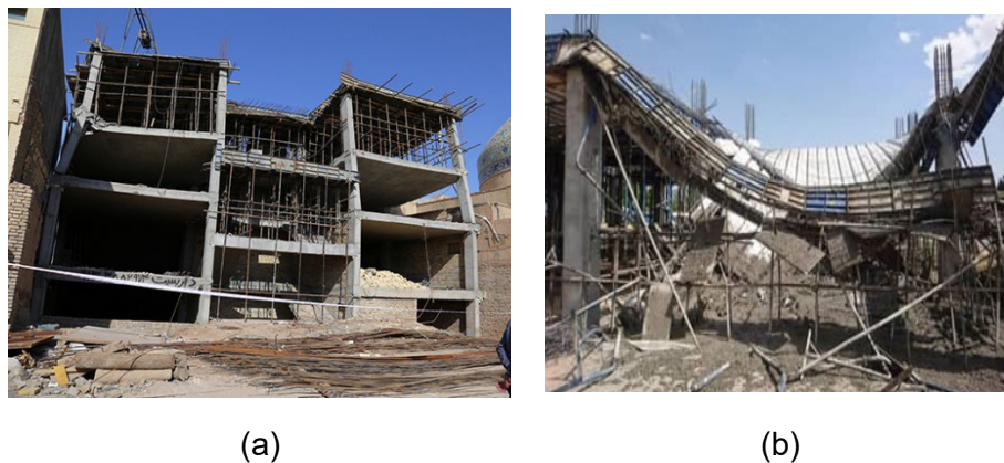
Fig. 5 - Construction operation issues at the construction site: (a) columns and beams reinforcements weakness; (b) reinforcement concrete slab failure
