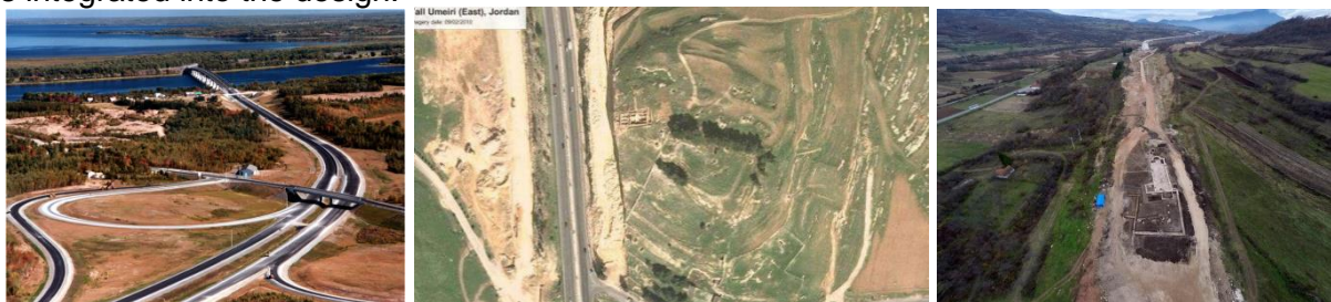
Fig.22 a) (left) Fredericton-Moncton highway (Canada)[48] b) (middle) Tall Ulmeiri (east), Jordan [49] c) (right) Kladence-Crnokliste (Serbia)
